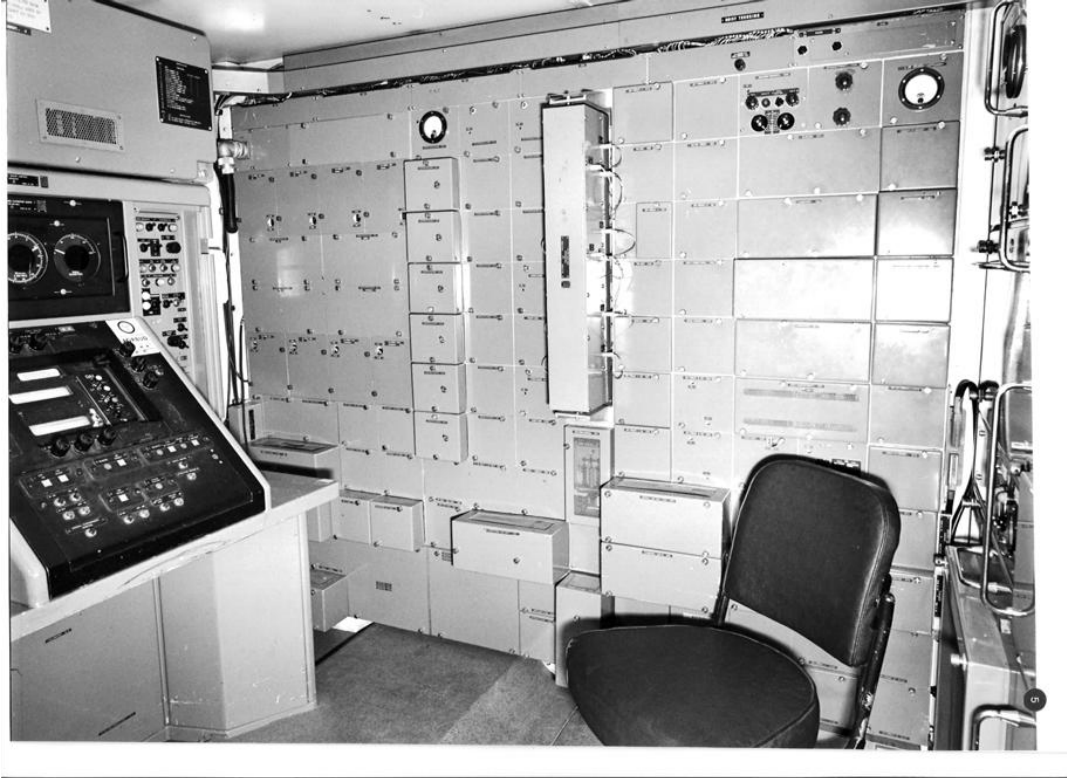
Radar Console D (left) and video unit C
