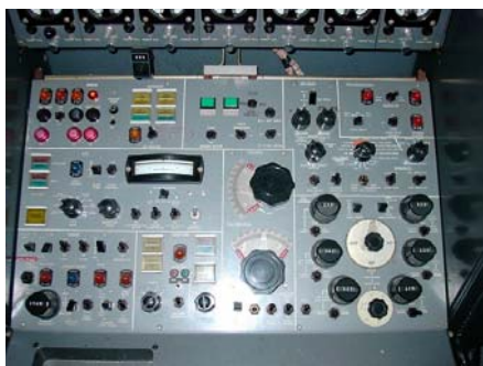
MOTE - Centre Control Panel
